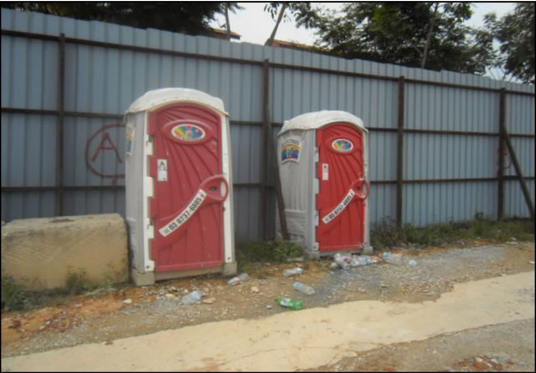
Modular self-contained septic tank system provided at site
